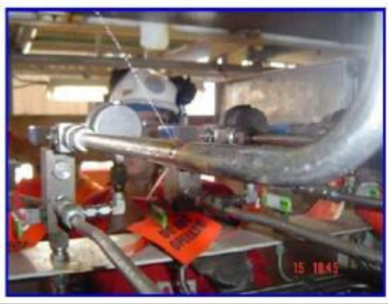
Figure 2 Pressure test leak within UTP
