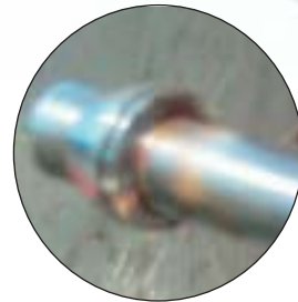
Close up of a corroded Back Ferrule in service
